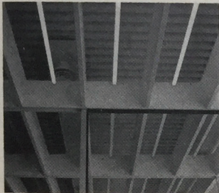
Louvered grid in Connecticut General Bldg. by Skidmore Owings and Merrill hides fluorescent tubes, ducts and diffusers; provides sound control
