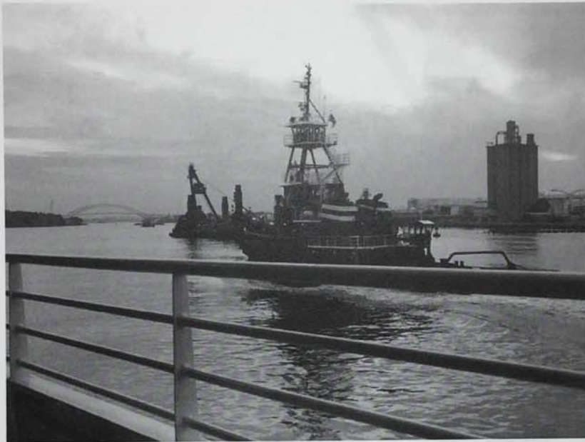
Dredging in the Kill Van Kull between Staten Island and New Jersey, under the jurisdiction of Matthew Baird Architects.
