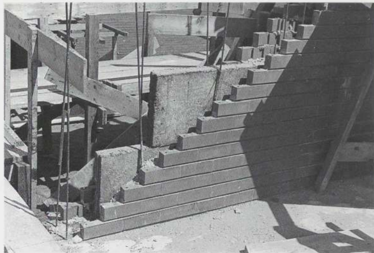
Figure 19: Frank Lloyd Wright. S. C. Johnson & Son, Inc. Administration Building, Racine. 1936–39. Exterior wall under construction
