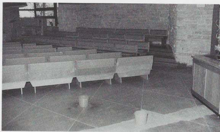
Figure 10: Frank Lloyd Wright. Unitarian Church, Madison. 1945–51. Interior view with buckets for collecting water
